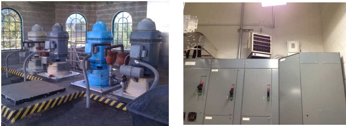
Figure 3-3 Photos of Existing RWPS (left) and MCC Room (right)
