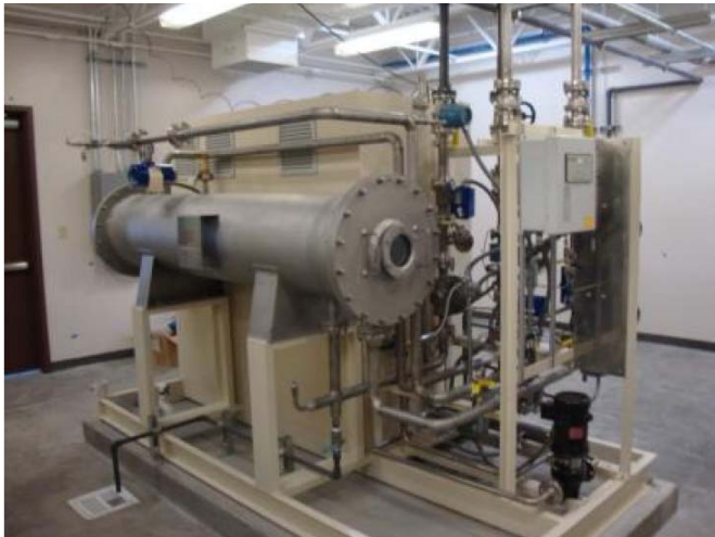
Figure 5-6 Ozone Generator Skid System
