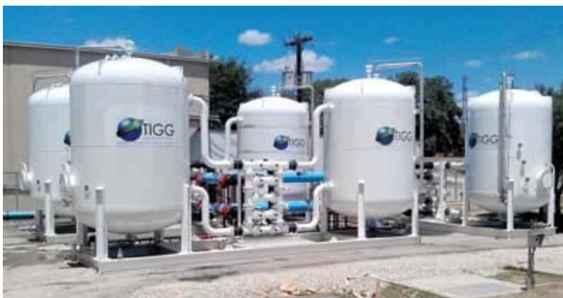
Figure 5-8 Pressurized GAC Contactors installed in San Antonio (photo courtesy of TIGG)
