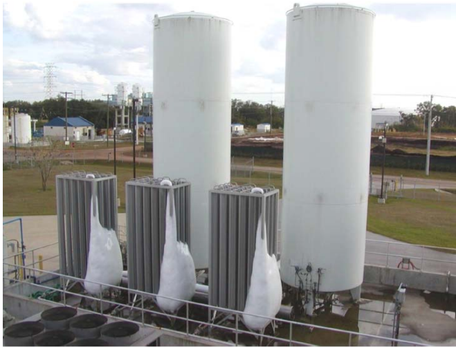
Figure 5-7 Liquid Oxygen Storage for Ozone Generation
